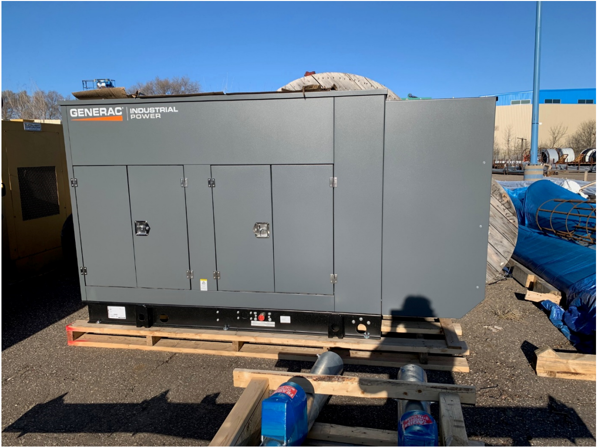
Well 2 Generator – Stored at the Killmer Electric Office
